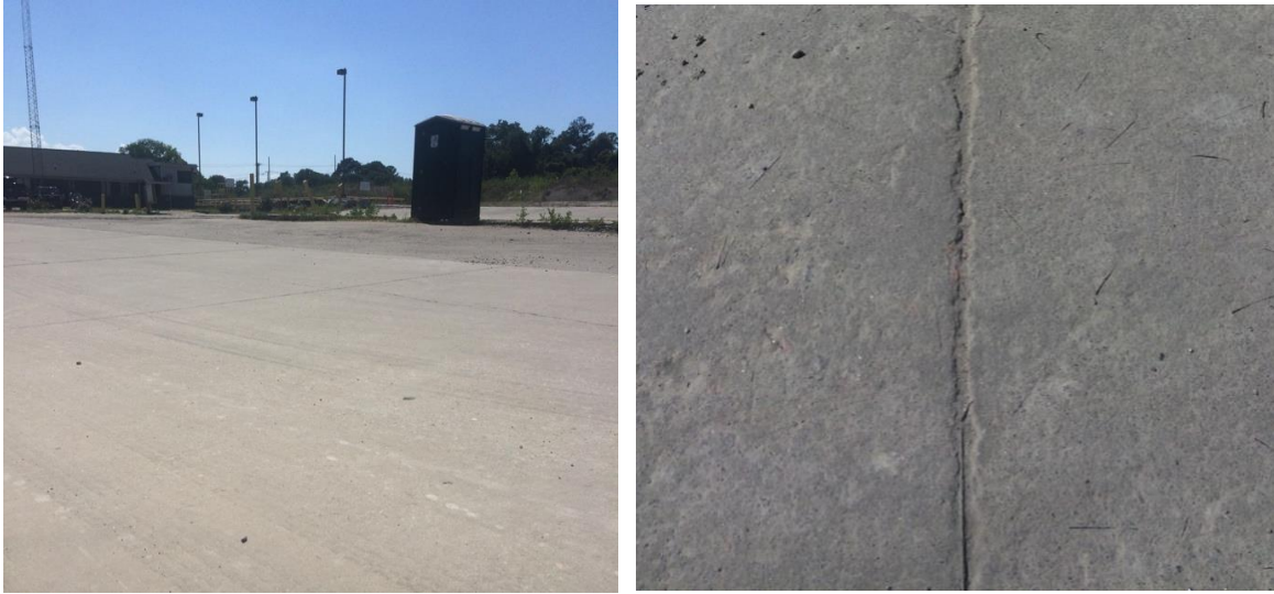
Figure 6. Pavement Condition after 8 Years
